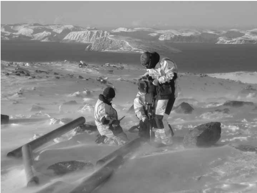
Figure 1 Foundation work in connection with site measurement campaign. Photo: Kjeller Vindteknikk, Norway.
