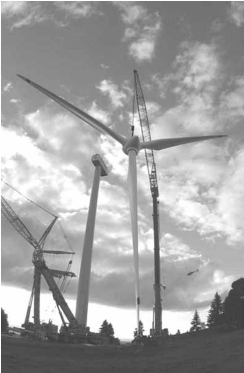
Figure 2 Installation of a 1.75-MW wind turbine on Mt. Crosin by Juvent SA.
