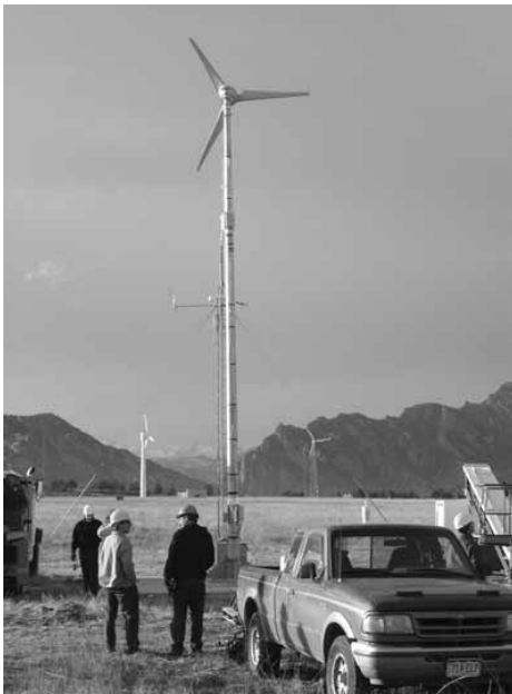
Figure 5 The Southwest Windpower Storm prototype turbine was installed at NREL in December 2004 for field-testing.
