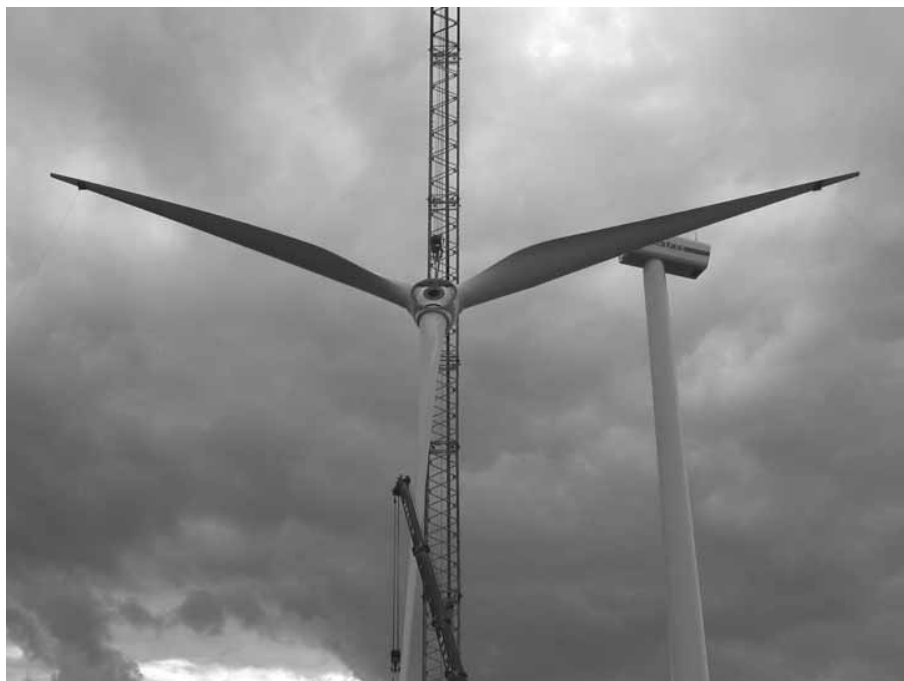
Figure 5 Vestas V80 2-MW turbines at FRI-EL's site in the Campania region.
