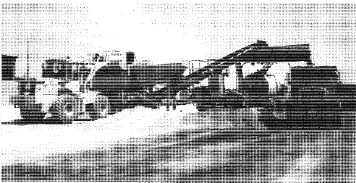
Figure 7.5 Cold-Mix Continuous Plant
