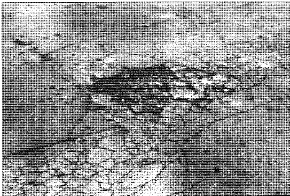
Figure 9.1 Deteriorated Asphalt Pavement and Candidate for Recycling
