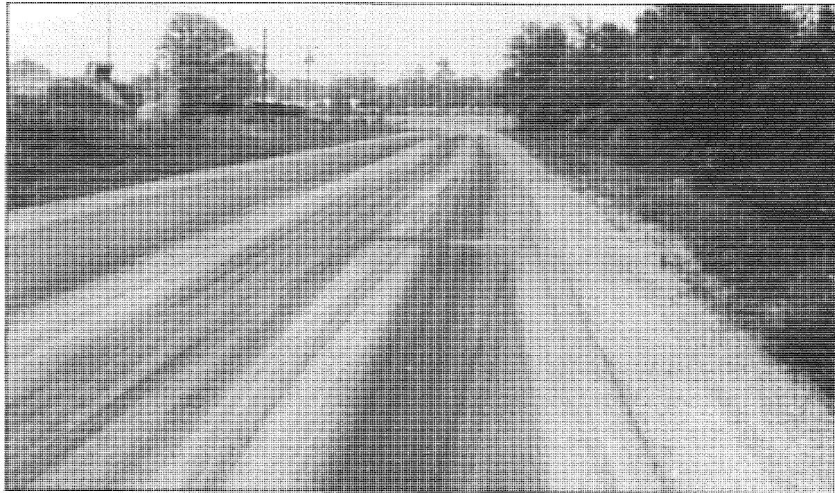
Figure 6.17 Loss of Cover Aggregate
